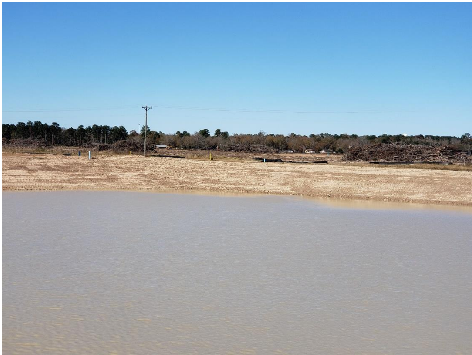
Portions of Detention Pond #1 Require Stabilization
