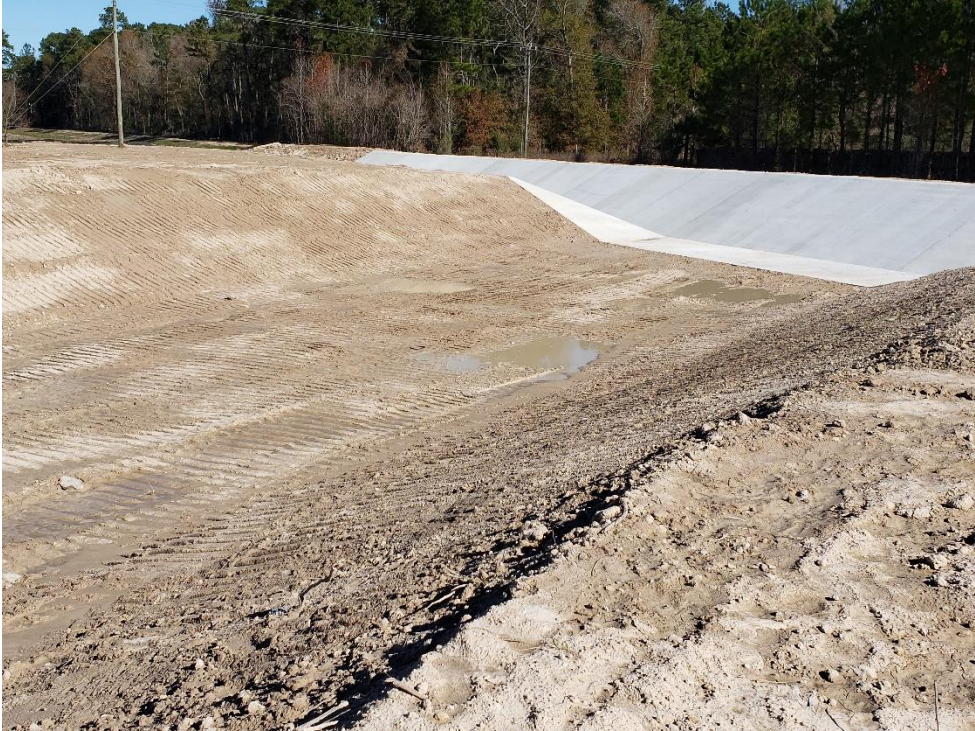
Overflow of Montgomery County Flood Control Ditch to Detention Pond #1
