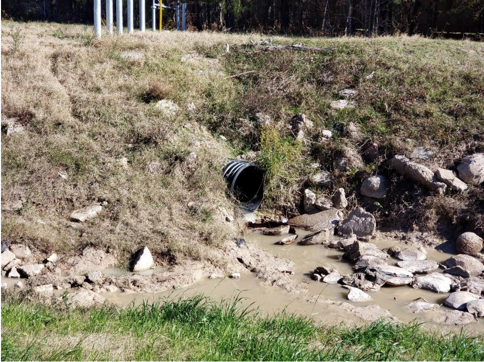
View of Outfall of Montgomery County Flood Control Ditch to Taylor Gulley
