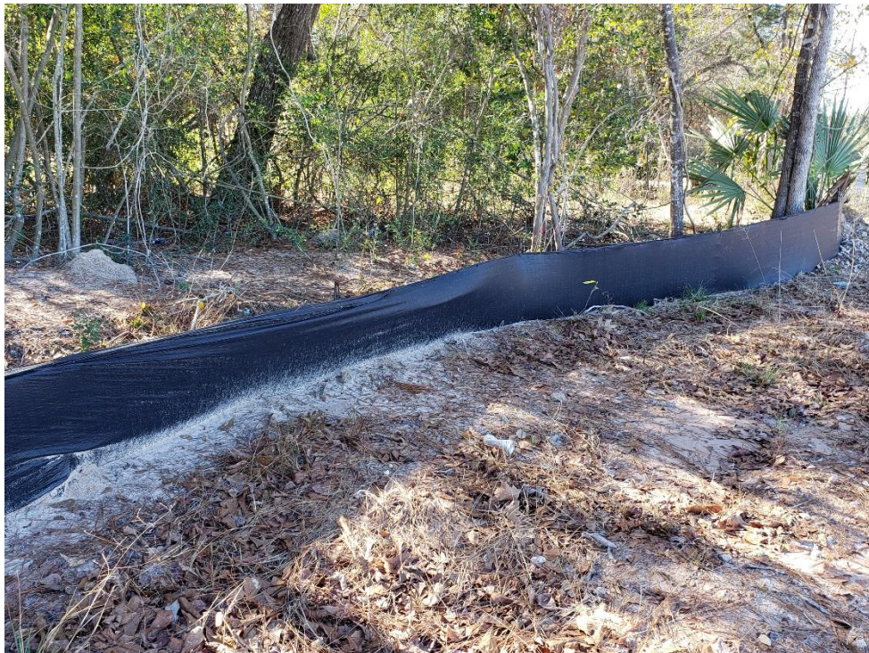
View of Silt Fencing in Good Repair
