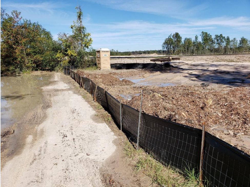
Well Maintained Silt Fencing
