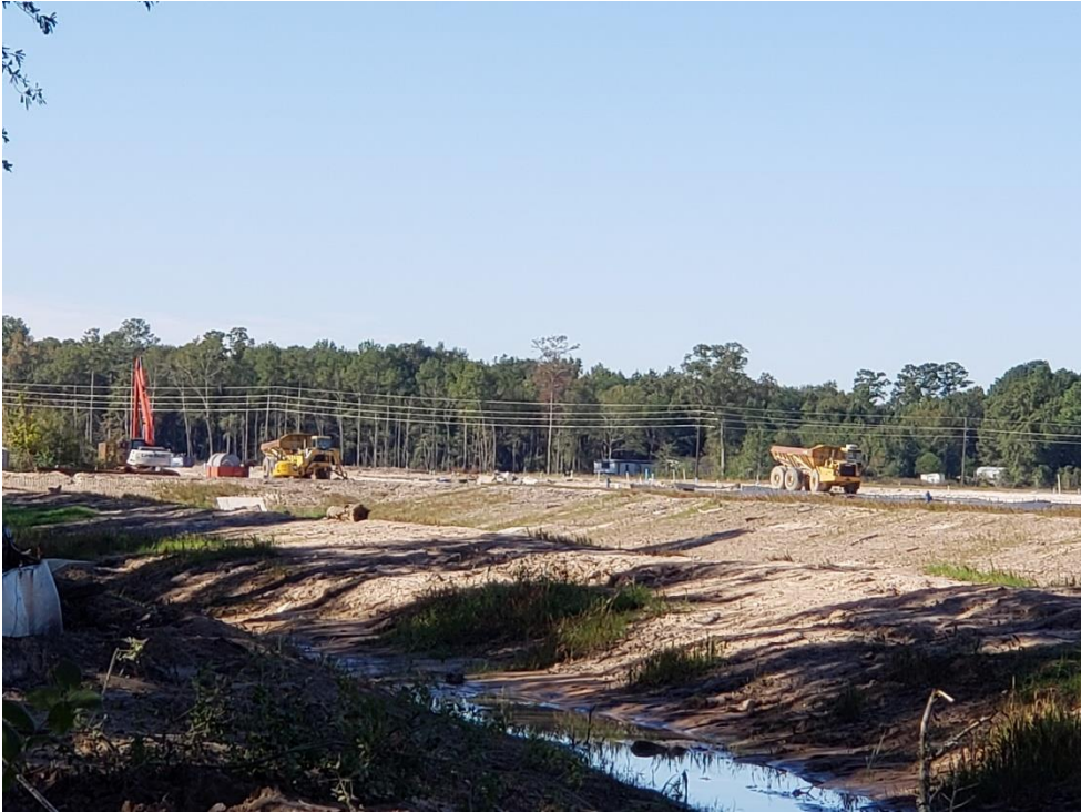
View of Idle Equipment Looking West
