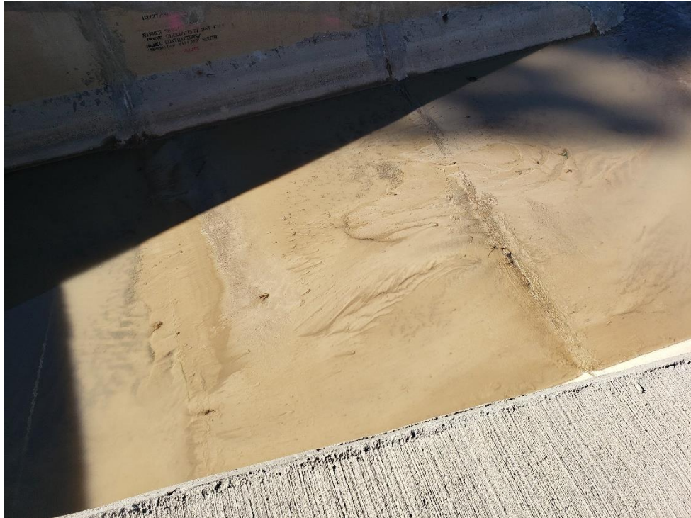
Shallow Sediment Accumulation in Outfall Structure
