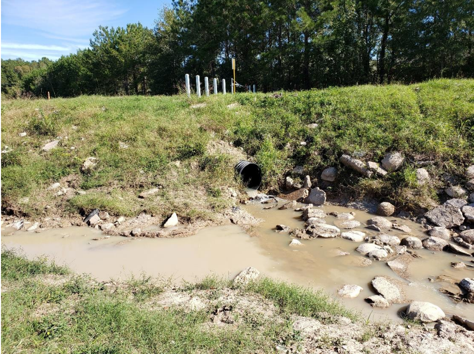
Discharge from Montgomery County Drainage Ditch to Taylor Gulley
