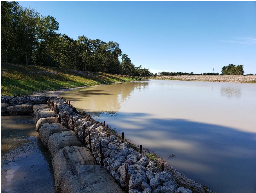
View of Detention Pond #1 Looking West Note: Some stabilization on south slope
