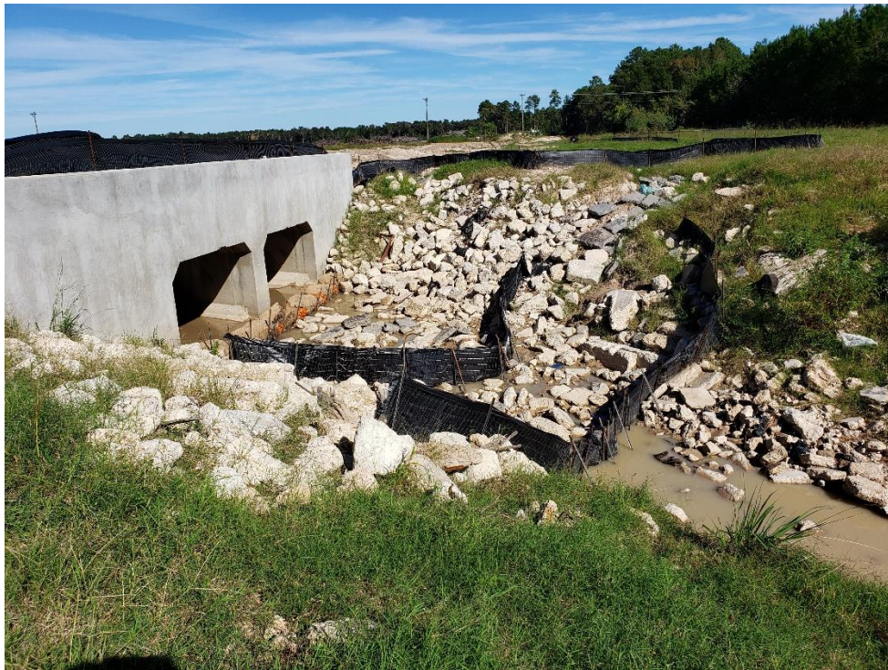
Detention Pond #1 Outfall Structure to Taylor Gulley Note: Hay bales and double silt fencing added
