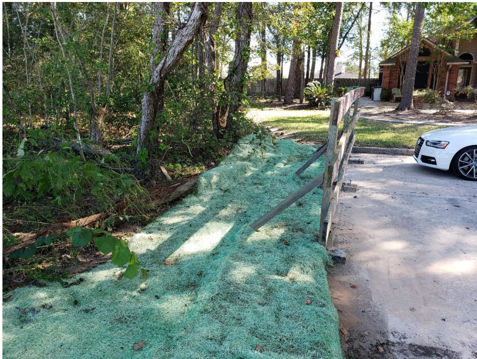
View of Village Springs Drive with Curlex Blanket Stabilization Note: Debris has been removed
