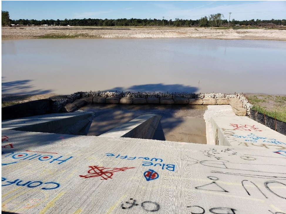
Detention Pond #1 Upstream Outfall Structure to Taylor Gulley Note: Hay bales have been maintained and secured
