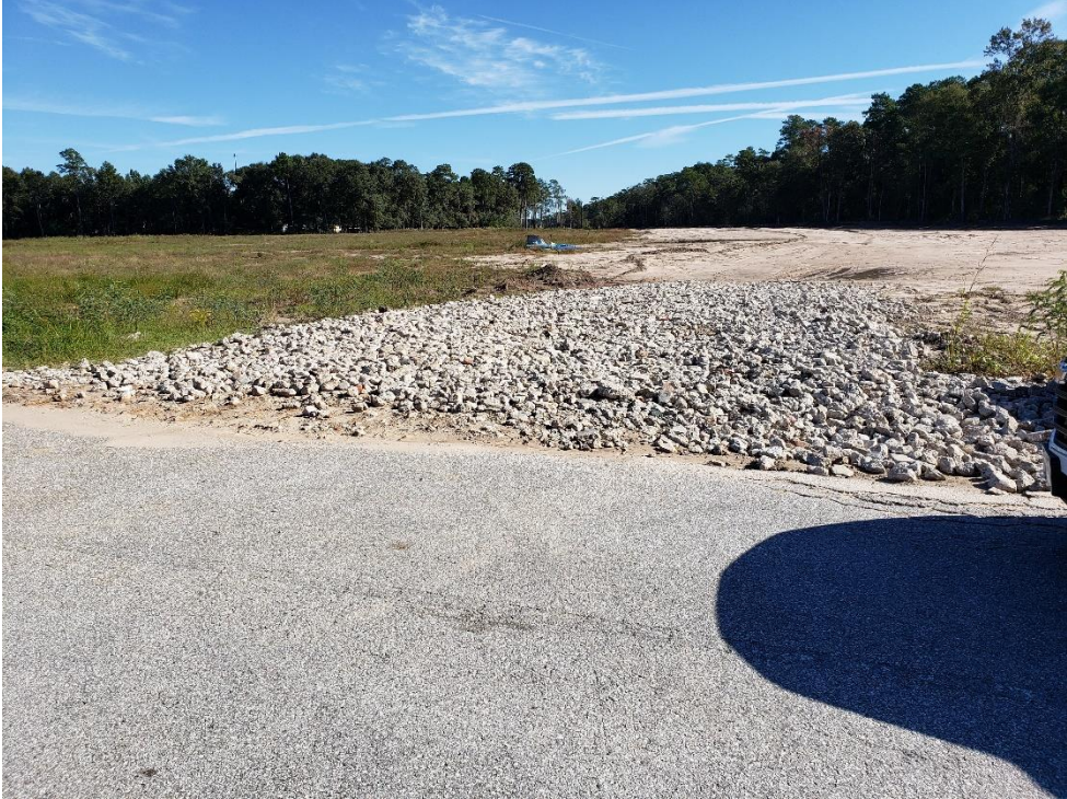
Construction Site Entrance on Woodland Hills Drive Note: Light sediment
