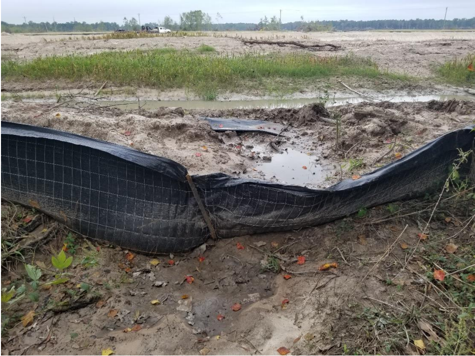
Silt Fence Requires Maintenance
