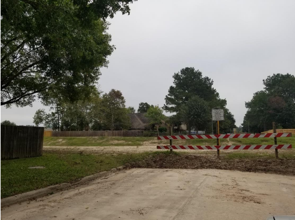
Creek Manor Drive Requires Sediment Removal and Stabilization
