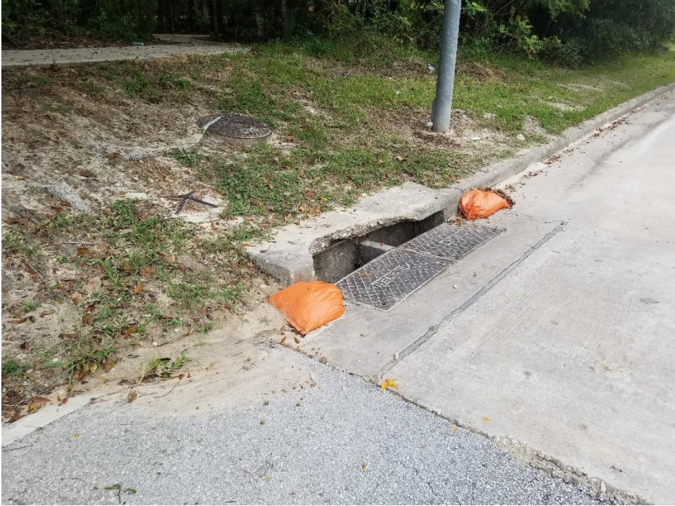
Inlet Protection with a Small Amount of Sediment
