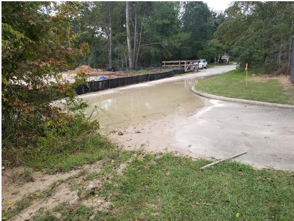
Fair Grove Drive, Ponding on Driveway to COH Well #6
