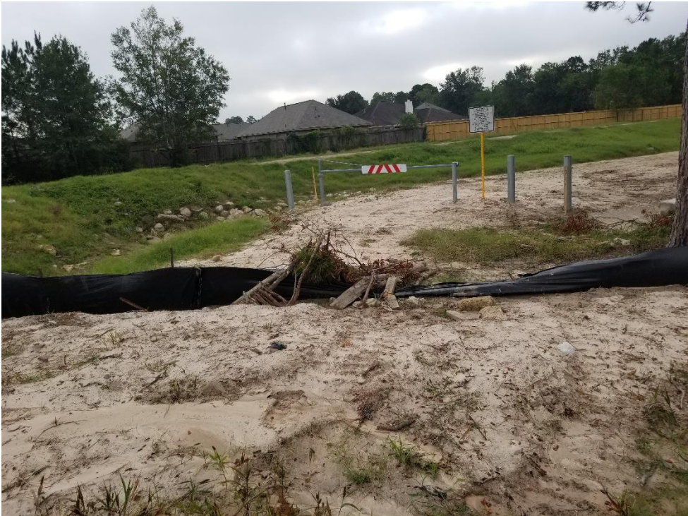
Silt Fence Near Outfall Structure Requires Maintenance
