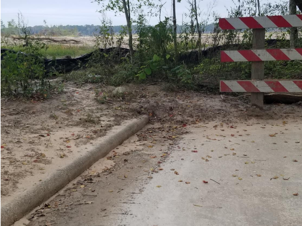
End of Village Springs Drive Requires Stabilization and Sediment Removal
