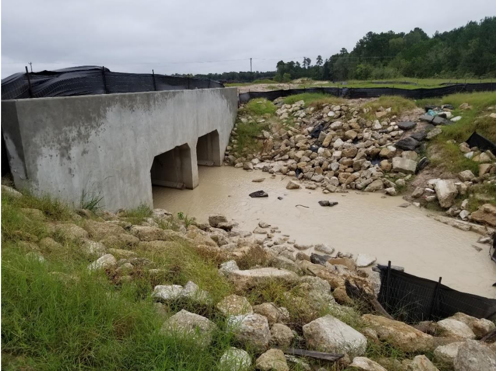
Hay Bales to be Added to Box Culvert Discharge to Reduce Sediment Migration
