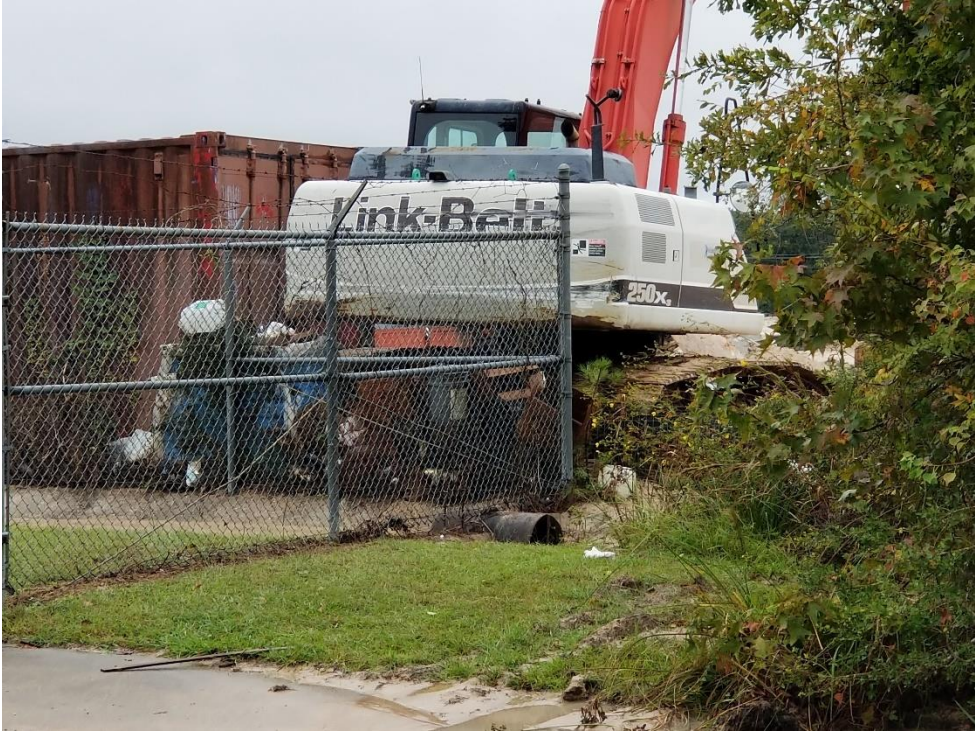
Trash and Debris at Temporary Staging Area
