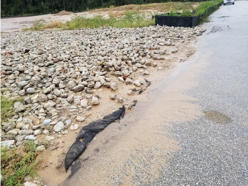
Light Sediment Washed from Construction Site Entrance
