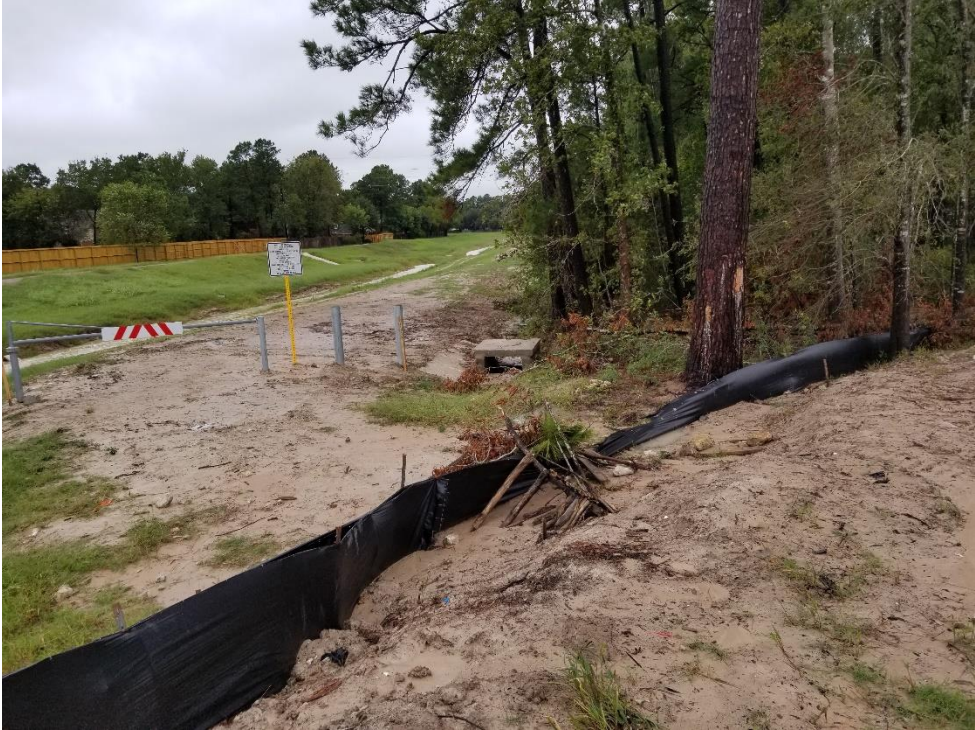
Silt Fencing Requires Maintenance
