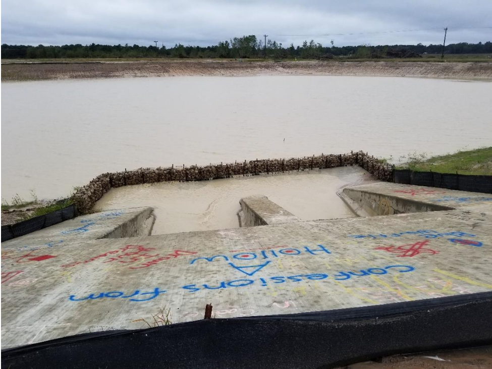
Upstream of Outfall Structure on Detention Pond #1 Note: Add hay bales behind rock gabions to reduce sediment migration
