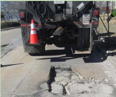
Punchout – NOW a pothole
