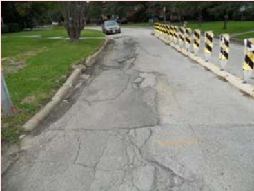
Localized Pavement Failure
