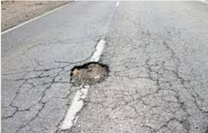
Pothole – NOW up to 25 ft 2
