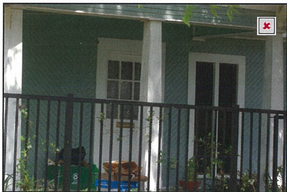
Siding applied in an incompatible herringbone pattern
