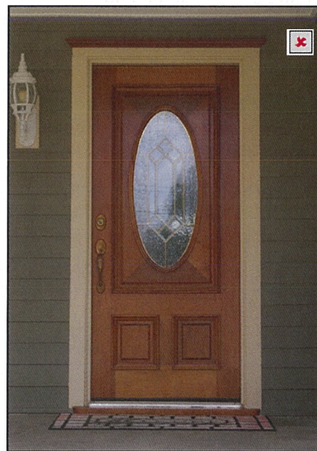
Incompatible replacement front door
