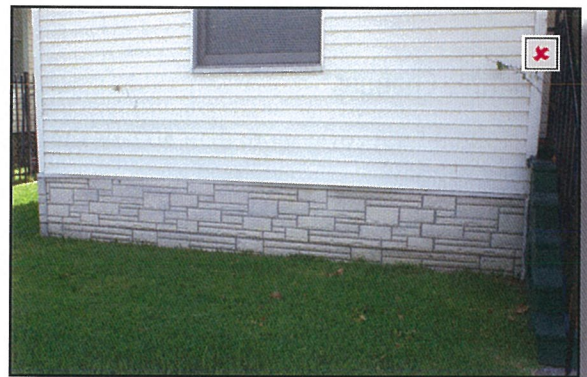
Incompatible faux stone foundation skirting
