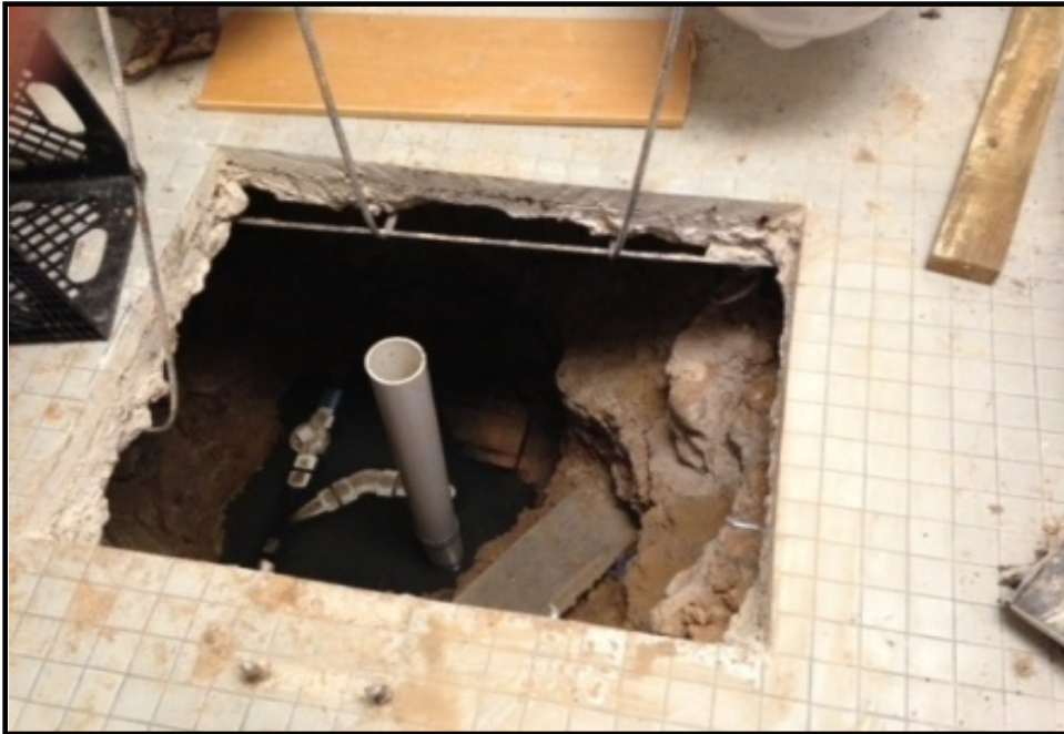
Recently discovered sink hole and recurring plumbing issues Foundation shift/settling near the employee rear entrance
