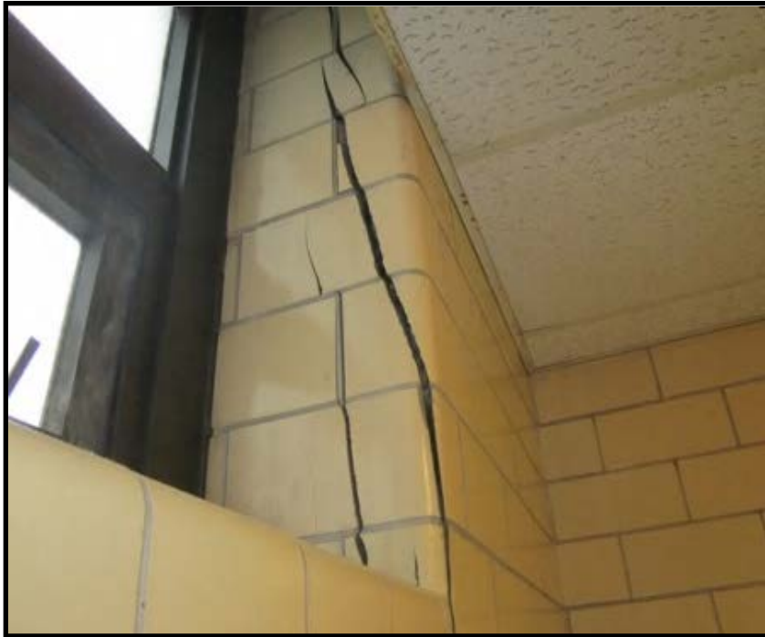
Cracks throughout the building indicate foundation problems
