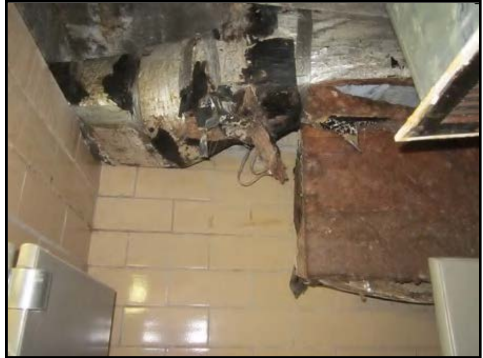
Mechanical and plumbing systems have numerous leaks and failures due to their age
